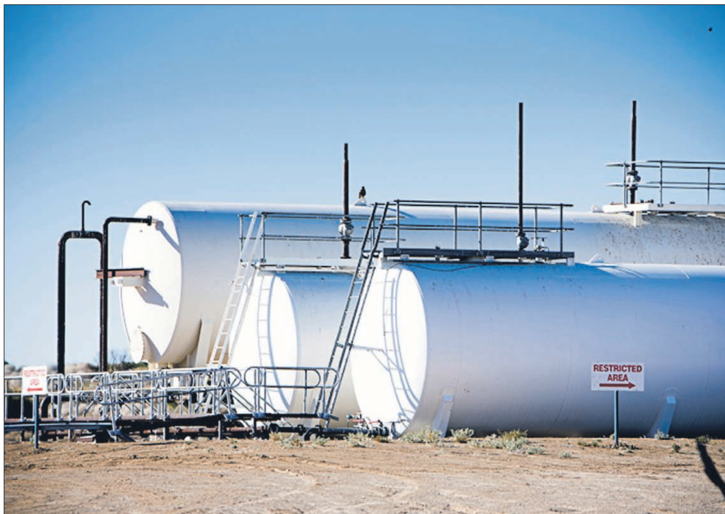
Crude oil separator at the Chiton oil field in the Cooper Basin
